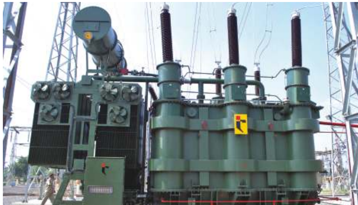
T&R's first 200MVA, 220/132/11kV Transformer supplied to MSETCL, Amravati substation was dispatched from Changodar Plant on 28th July 2009. The transformer reached the site on 10th August 2009. The erection work started on 26th November 2009 and was commissioned on 12th December 2009.
