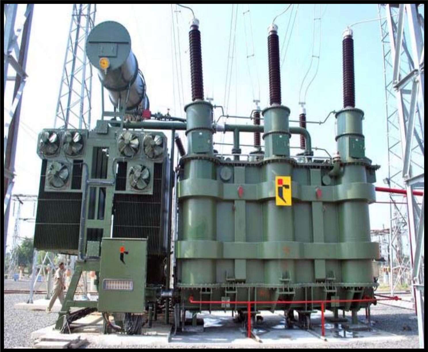
This is the highest rating transformer (in terms of MVA) successfully commissioned by TRIL
